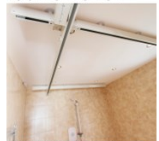
Small H-System in bedroom ensures client has full access
